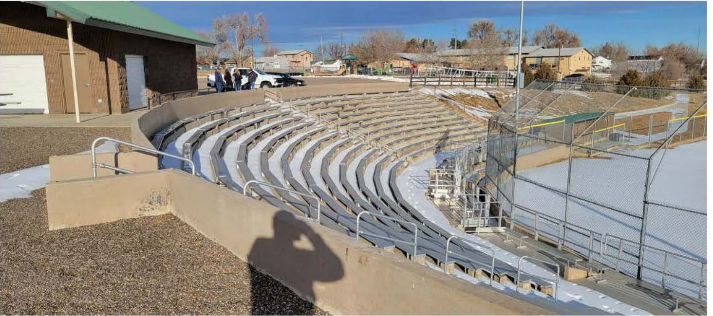
FORBES 2 - Existing bleachers and upper retaining wall (potentially beginning to collapse and slide downhill).
