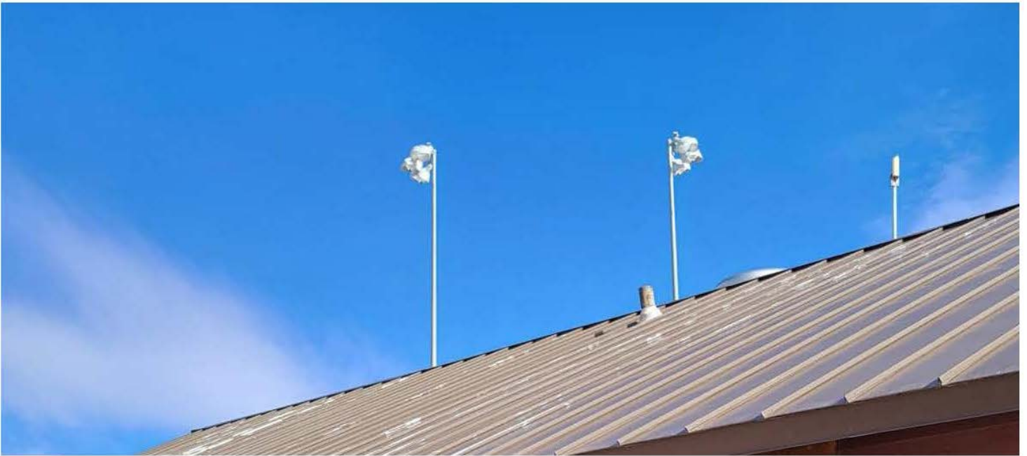
TWIN RIVERS 1 - Original sports field lighting to be replaced with LED fixtures.
