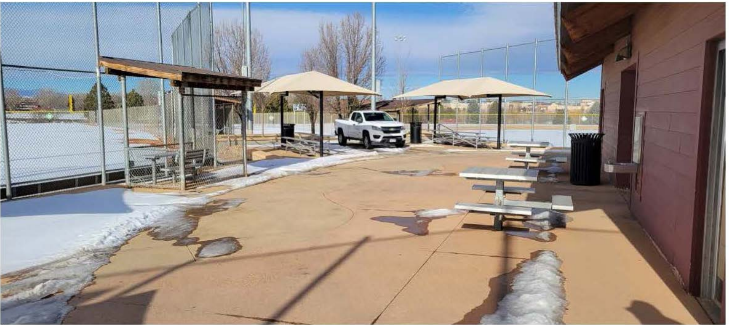
TWIN RIVERS 3 - Central spectator area in need of minor maintenance repairs; background fields to be considered for conversion from natural to synthetic turf.
