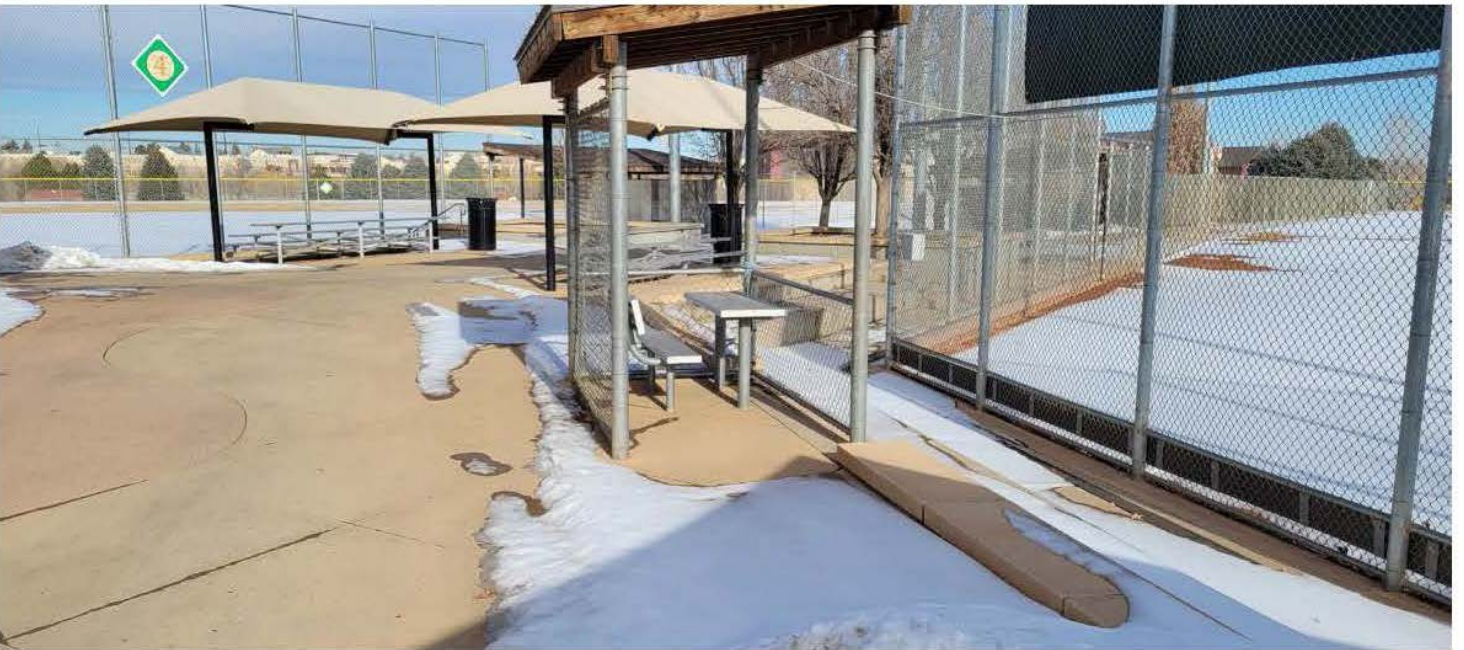
TWIN RIVERS 4 - Central spectator area in need of minor maintenance repairs; background fields to be considered for conversion from natural to synthetic turf.
