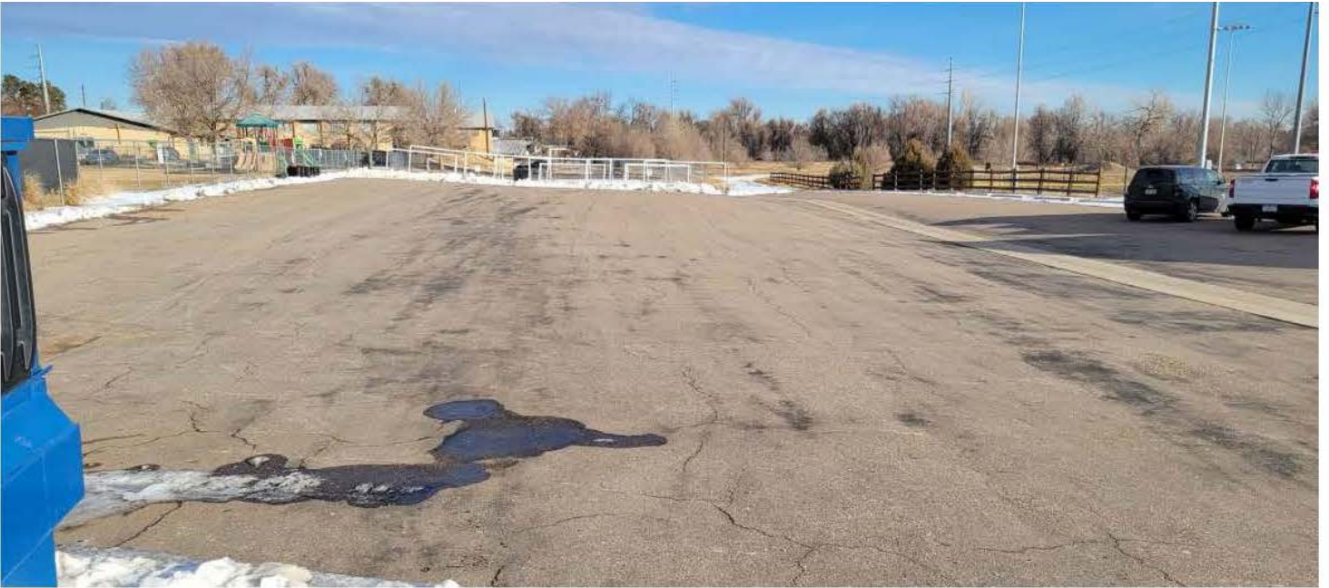
FORBES 3 - Existing southern parking lot in need of repavement.
