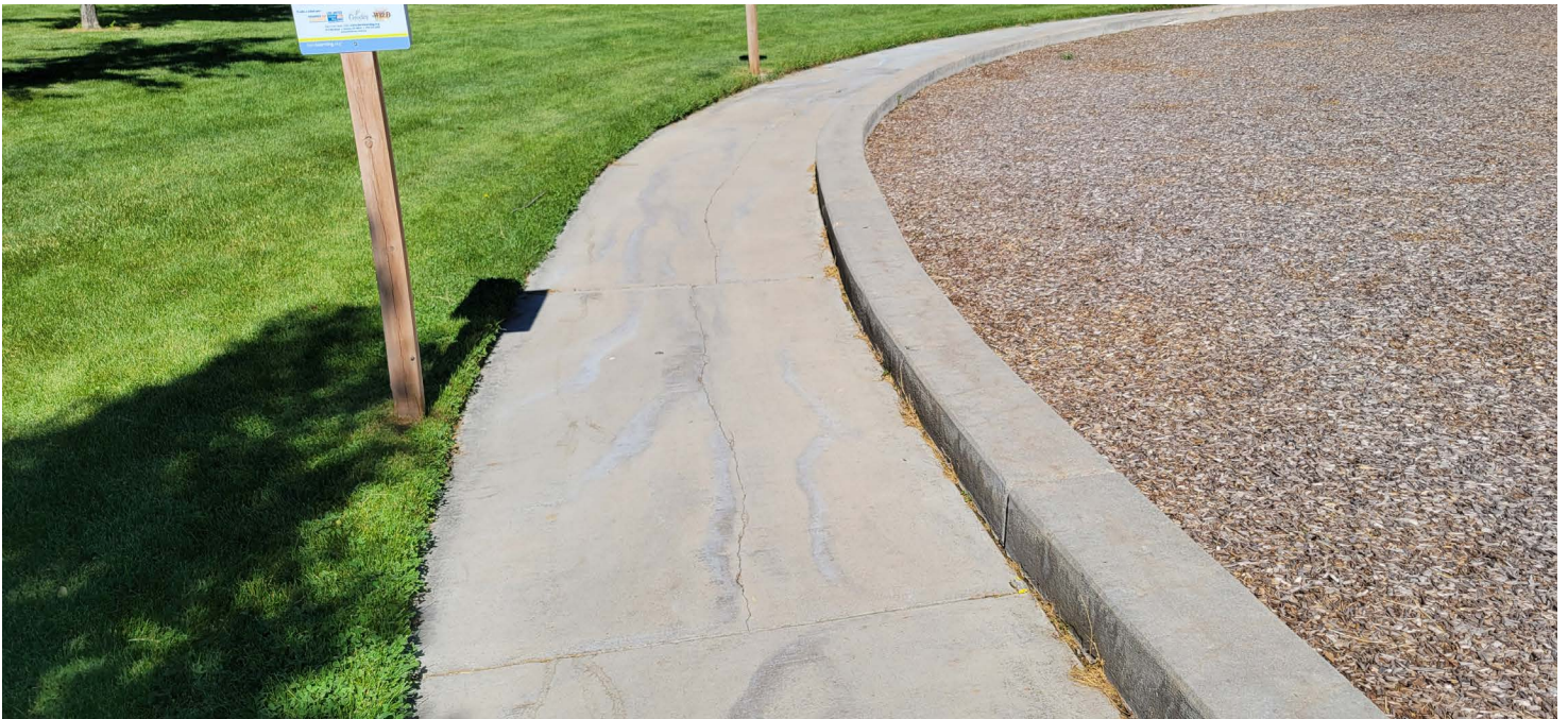
BITTERSWEET 6 - Example of cracked sidewalk near western playground area.
