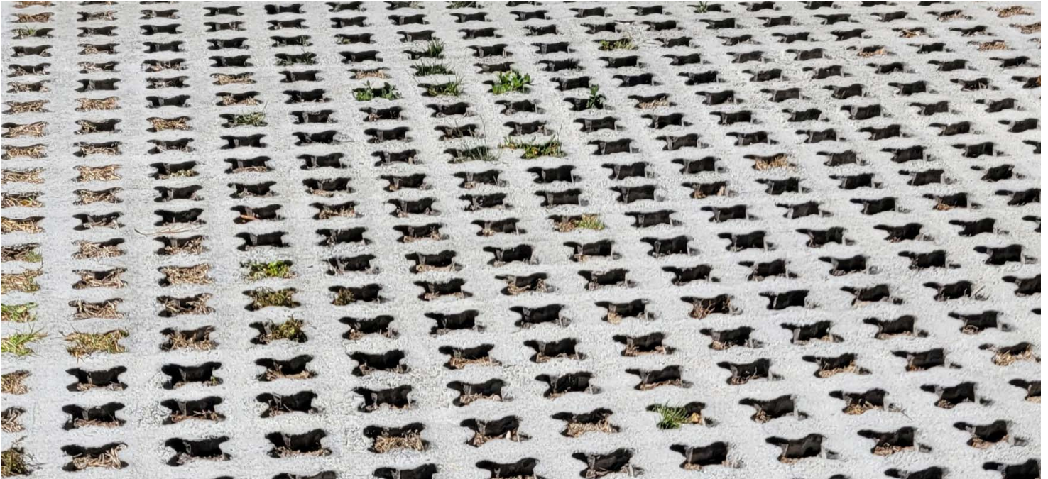
BITTERSWEET 8 - Existing "Grasspave" area lacking turf.
