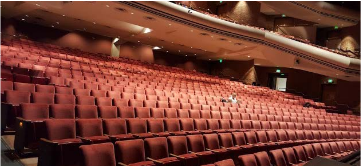
UCCC 2 - Theater seating in need of upgrade.
