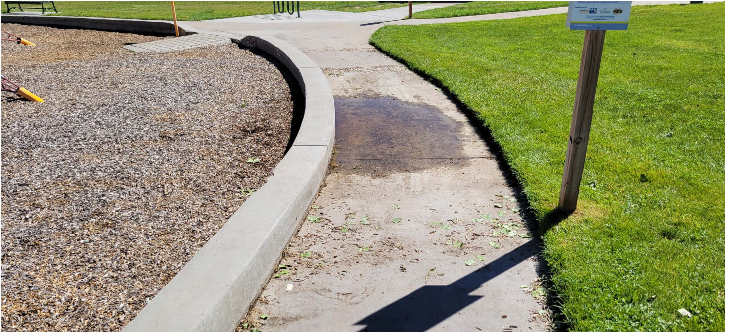
BITTERSWEET 7 - Example of ponding on sidewalk near western playground area.
