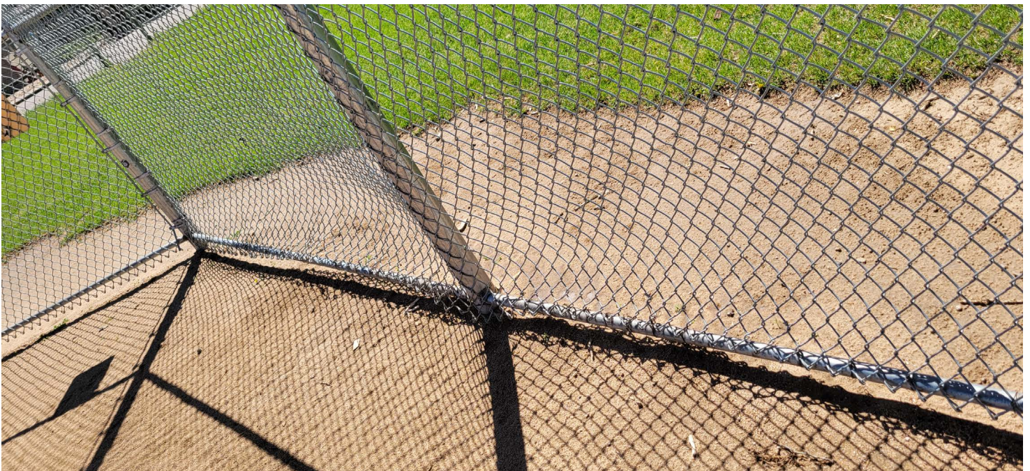
SHERWOOD 4 - Worn backstop fencing in need of replacement.
