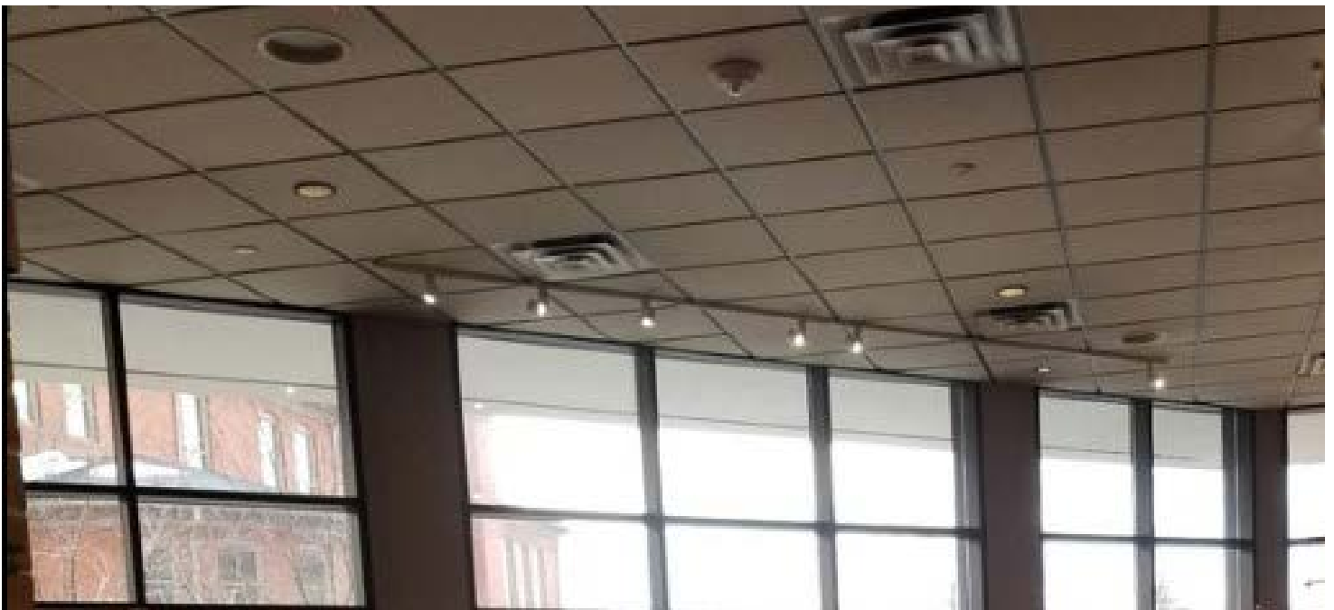
UCCC 3 - Water-damaged lobby ceiling in need of repair.
