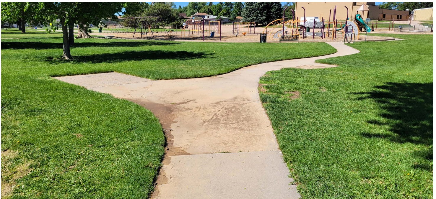
SHERWOOD 2 - Excess pavement (to left of sidewalk) near playground.
