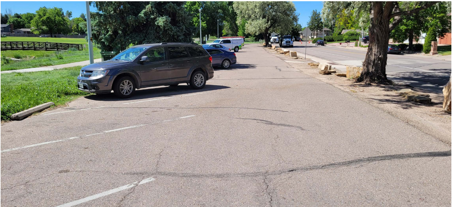
BITTERSWEET 5B - Existing western parking lot in need of repavement.
