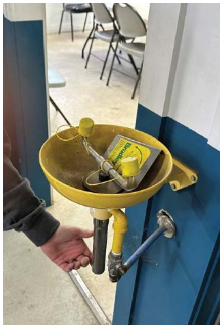
Figure 138: Eyewash station lacks proper drainage
