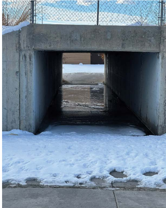
Figure 141: Tunnel under road lacks proper drainage:
